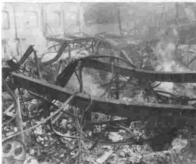
Fig. 1. Collapse of structural steelwork in severe fire.
