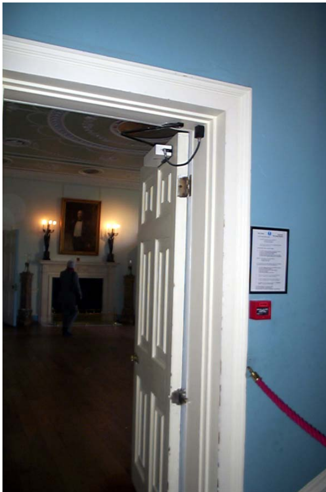
Figure 13 Fire door with hold-open device released by fire detection
