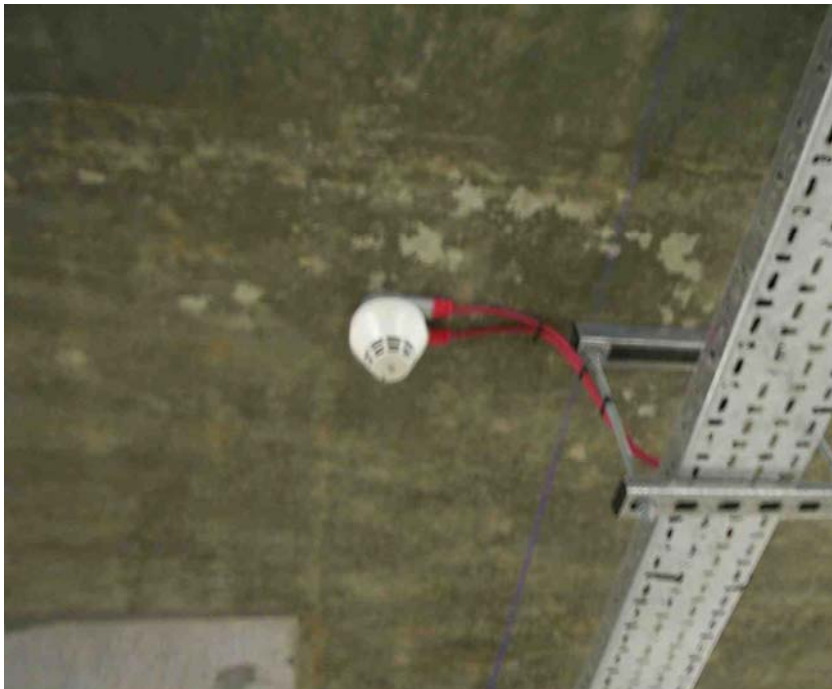
Typical fire detector and sounder for 2-level basement car park
