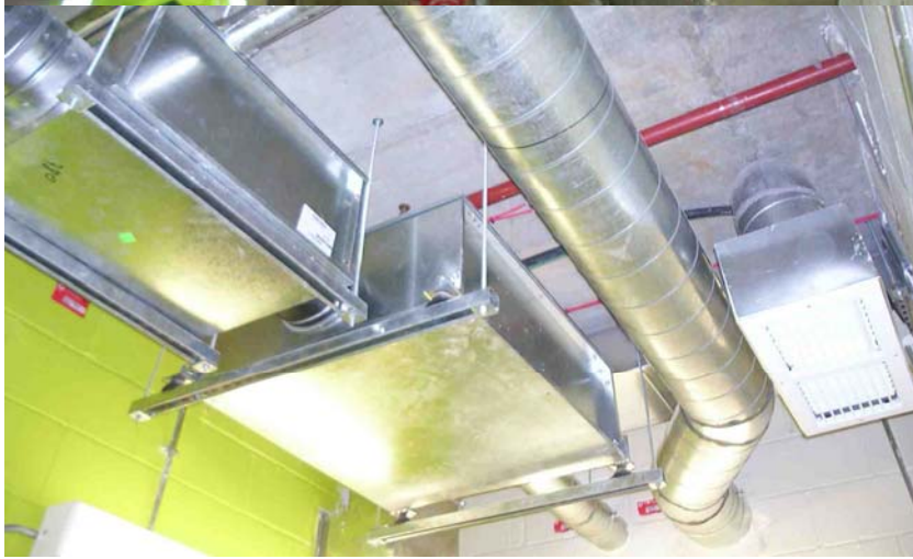
Exposed air handling plant on soffit in Community Focus
