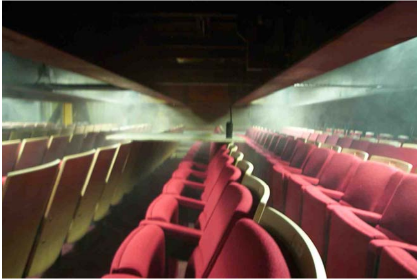
Seat store with smoke test on VESDA aspirating detection system in progress. Small fire is in bin resting on board on top of seats (centre of picture)
