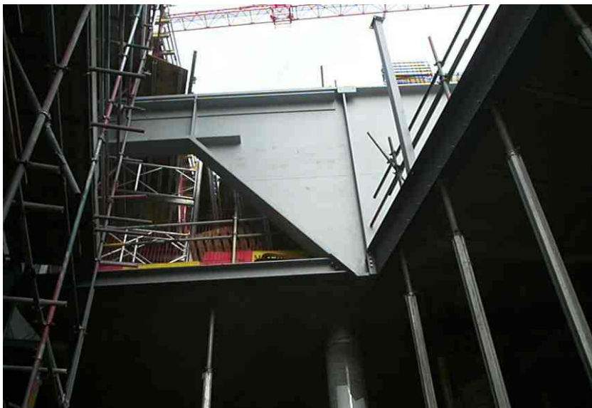
Part of massive storey-high steel plate girder acting as load transfer structure in the Arts Centre
