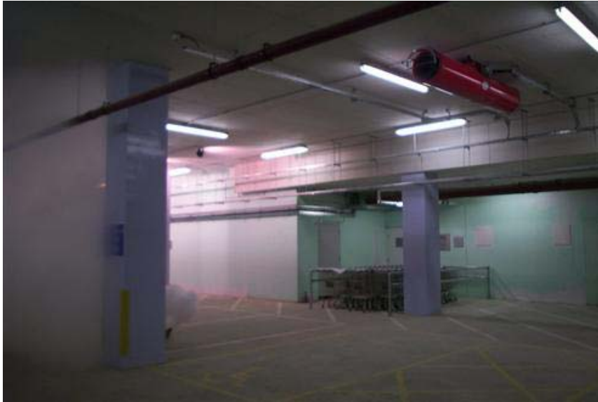
Top right hand side is red jet fan mounted below ceiling – one of roughly 30 fans used for smoke and vehicle fume removal. System avoids need for ducting.
