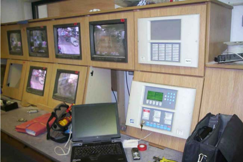
Control room monitors and fire control panels during commissioning
