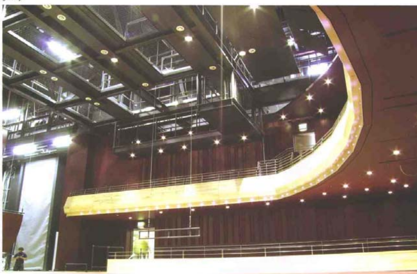
Pentland theatre lighting installation
