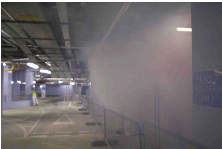
Part of smoke 'corridor' formed by PSB jet fans after they were switched on by detection system.
