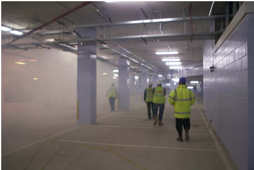
Smoke test in basement car park. Picture shows smoke logging before smoke control fans switched on.
